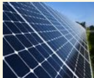
On-site Solar PV
