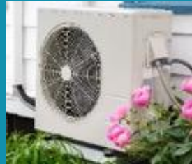
Air source heat pumps
