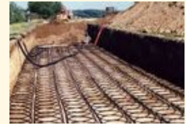
Ground source heat pumps
